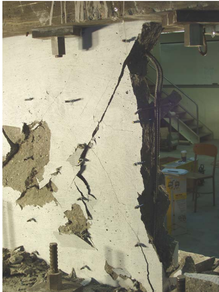
Axial load failure
