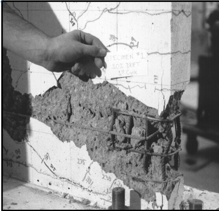
Rebar Buckling at Wall Boundary
