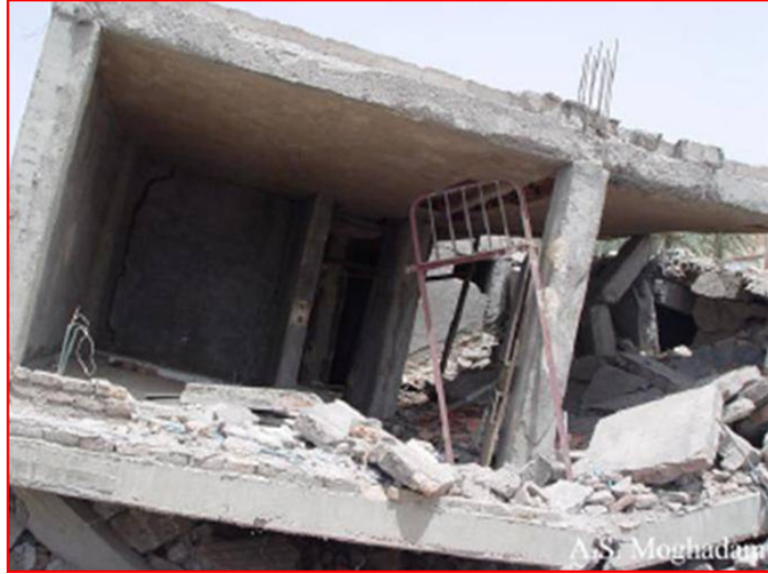
Fig. 1. A building damaged in Bam (2003) earthquake.
