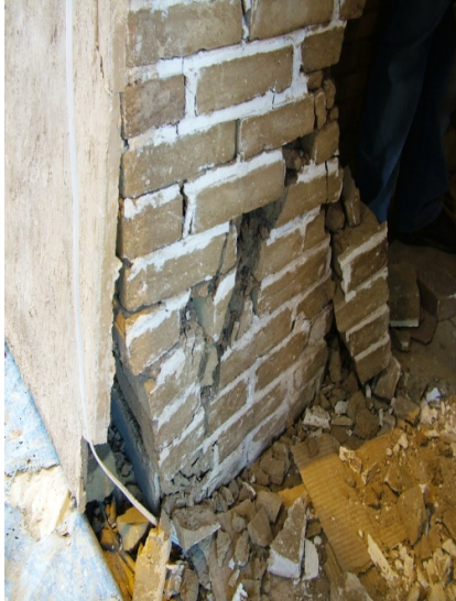
Fig. 10. Shear cracks at the base of door.
