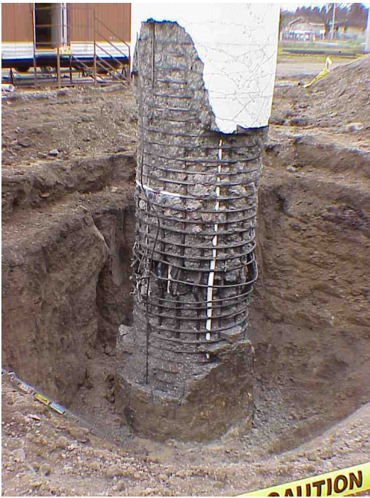
Fig. 2.- Plastic hinge below ground.
