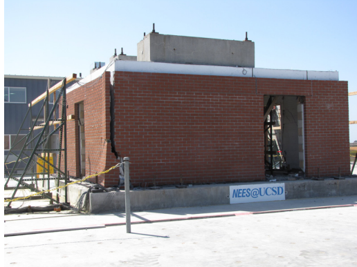
Fig. 4. Reinforced concrete masonry building, showing damage after the fifth incredible earthquake.
