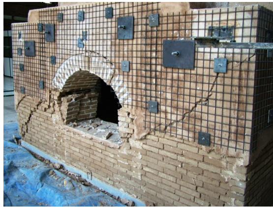
Fig. 12. Shear-due-to-torsion crack at eastern wall.
