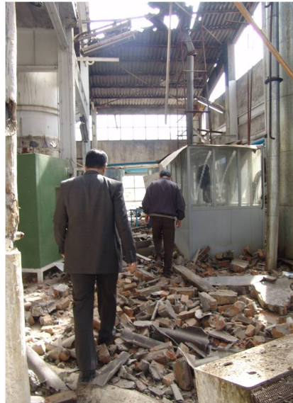
Fig. 2. Damage to non-structural elements in Silakhor (2006) earthquake.
