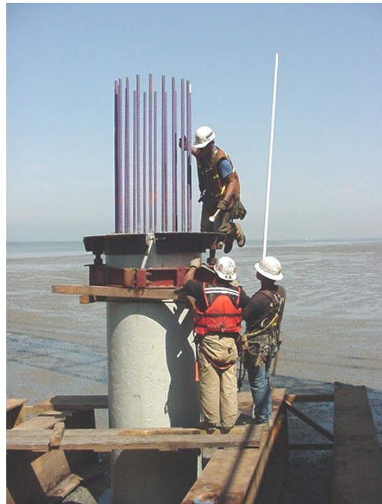
Fig. 8. Collar placed at top of column to support pre-cast bent cap beam.
