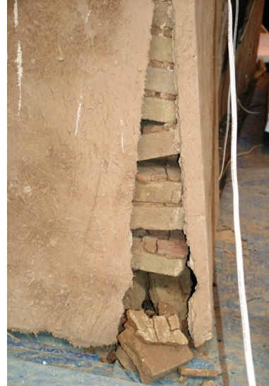
Fig. 11. Shear cracks at the corner.
