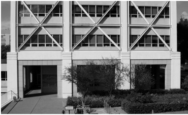
ABOVE: South entrance to University Hall displays soft story.
