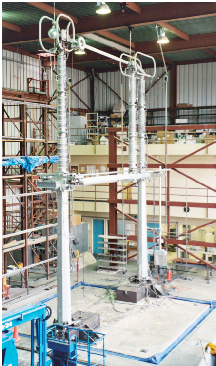
Fig. 1 550-kV switch in the closed position mounted on supports
