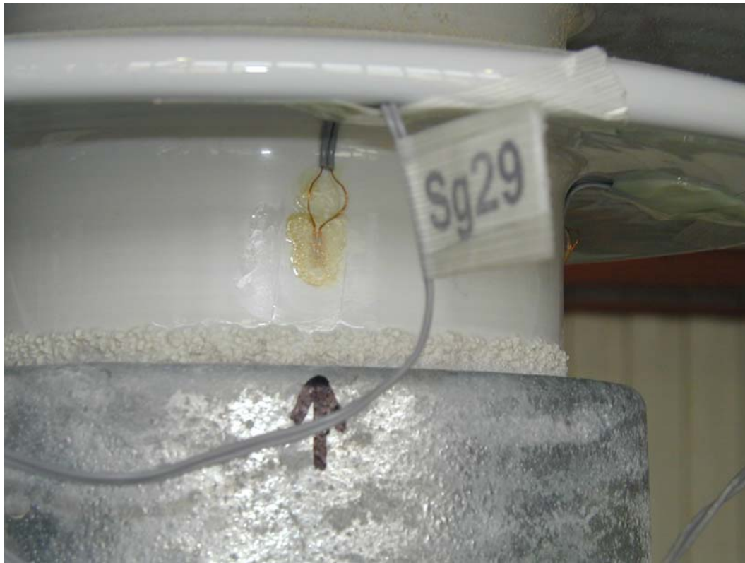
Fig. 2.9. Sample of typical strain gage installation on insulator post.
