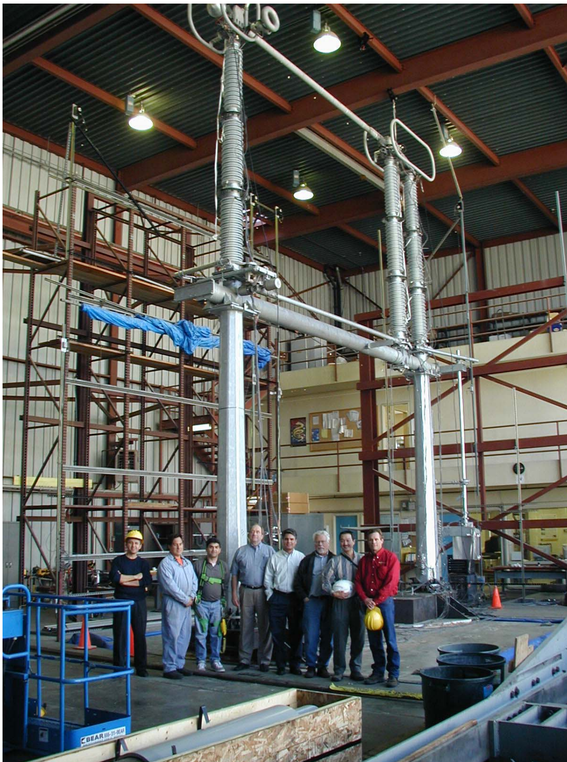
Fig. 2.2. Configuration 1: support-mounted configuration of switch (main blade closed).
