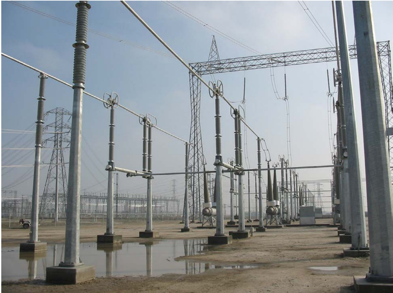
Fig. 1.1 Typical field installation of 500-kV disconnect switch consisting of 3 poles.
