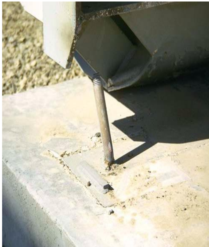
Figure 1.1. Overturned electrical equipment at Sylmar Converter Station damaged during the 1971 San Fernando earthquake (top), and a detail showing the failed back-left restrainer (bottom). Photos taken from the Steinbrugge collection, NISEE, University of California, Berkeley.
