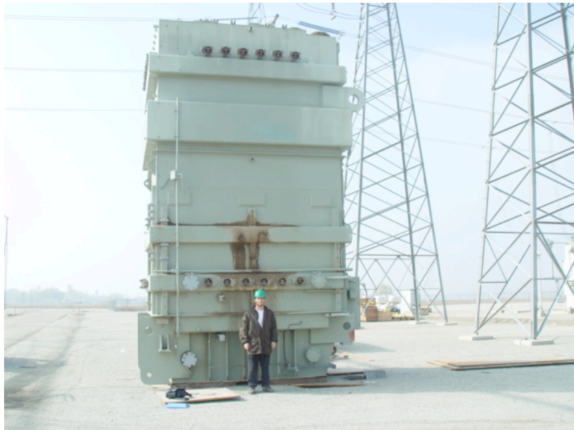
Figure 2.1 - 525 kV Transformer A.
