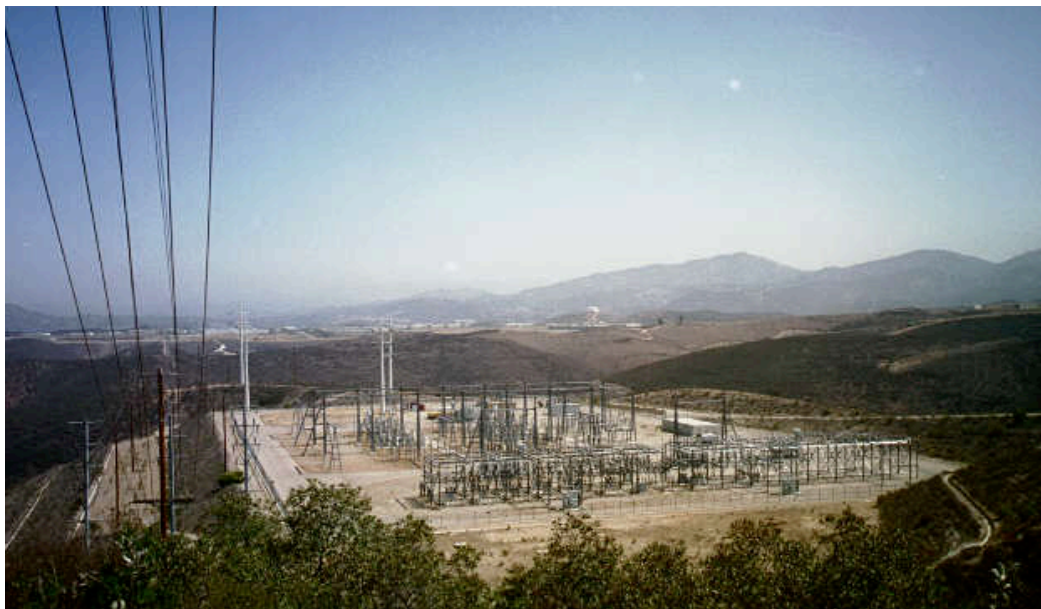
Figure 1.1 - Typical Electrical Substation.
