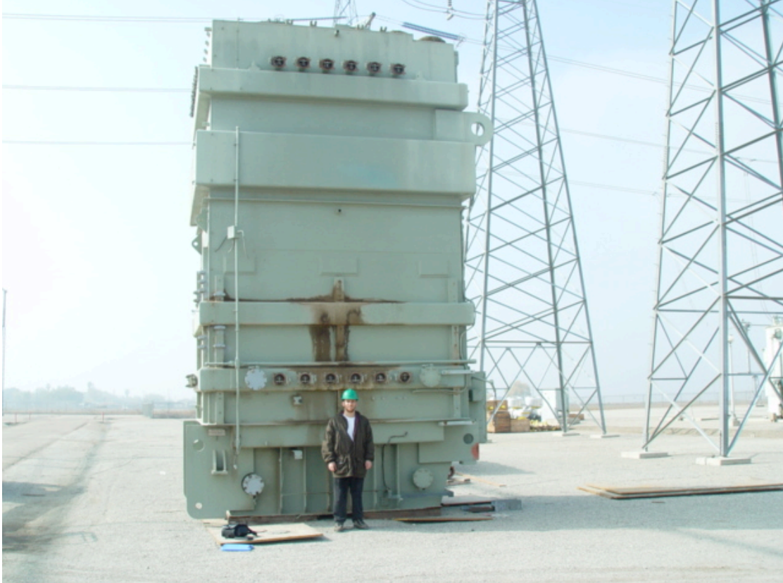
Figure 5.3 - 525kV Transformer A Test Specimen.
