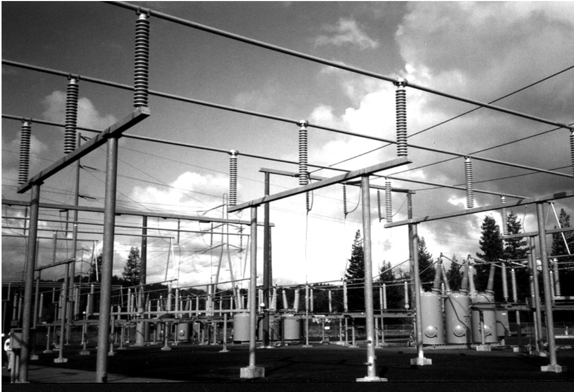
Figure 2.5 A 230kV bus support in service (Courtesy: PG&E)
