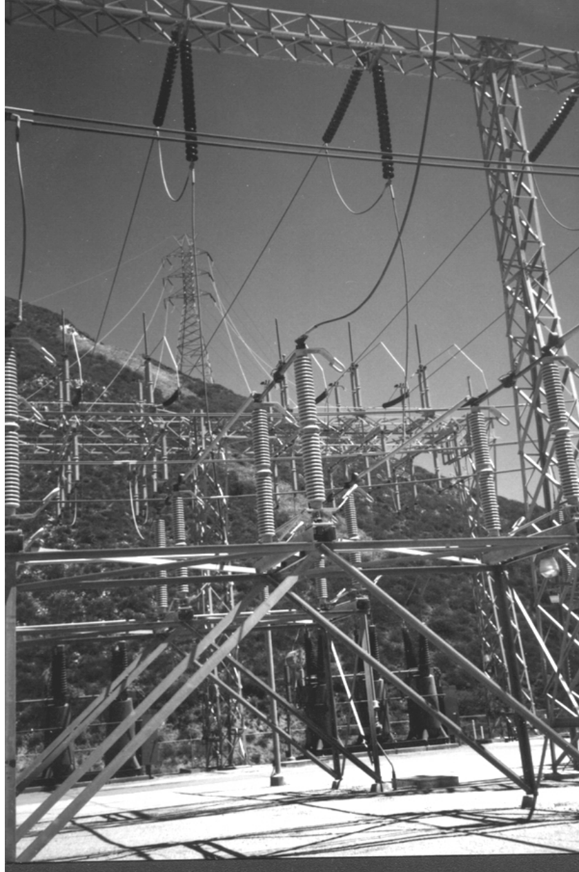
Figure 2.3 A 230kV disconnect switch in service (Courtesy: PG&E)
