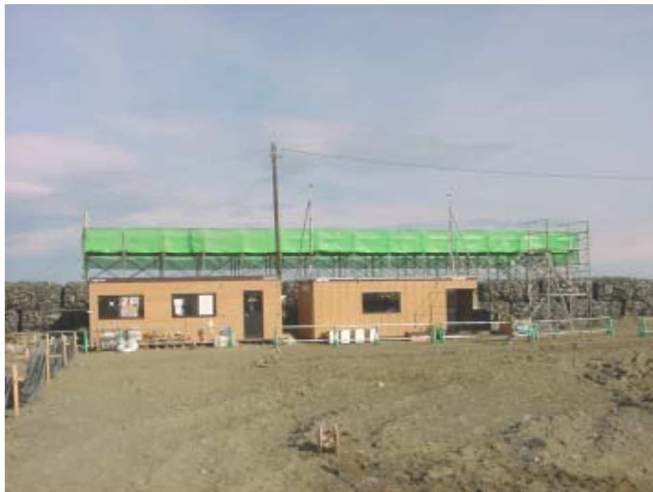
Figure 26 – Monitoring center trailer
