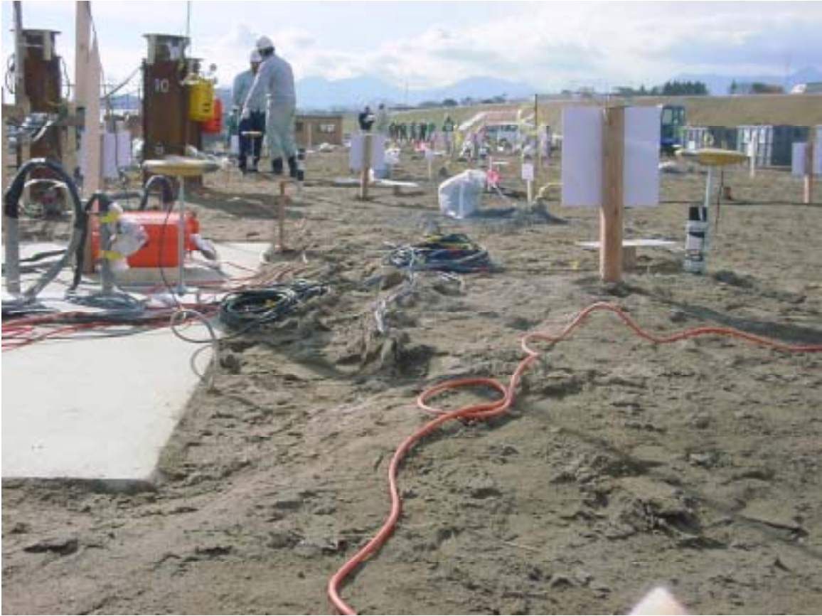
Figure 12 – Units 1A and 1B, November Test
