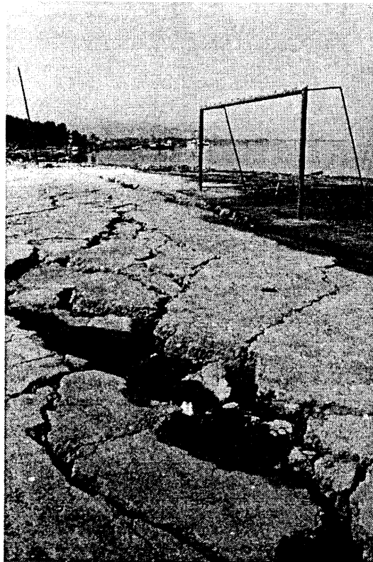
Figure 5-74: Extensive cracking in the Soccer site due to lateral spreading
