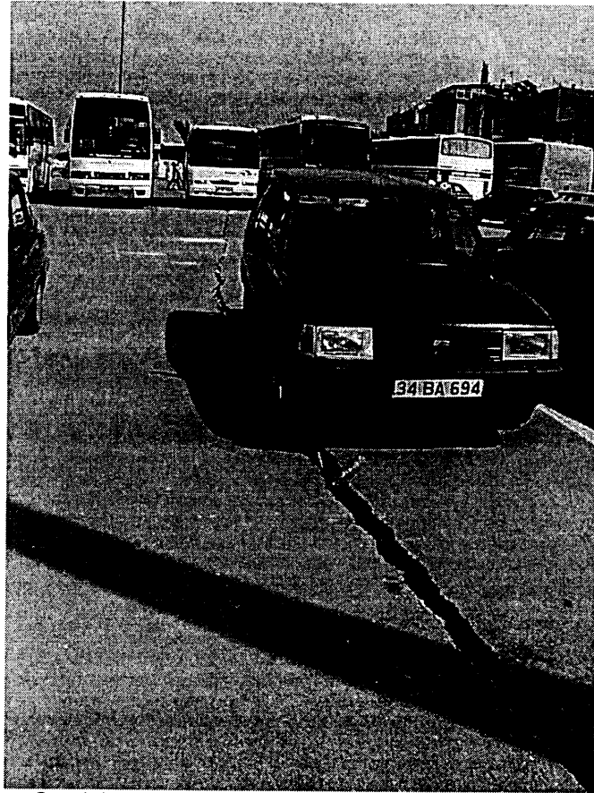
Figure 5-80: Crack in parking lot south of pier for ferry terminal at Yalova Harbor
