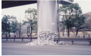
Failed bridges due to column failure from previous earthquakes
