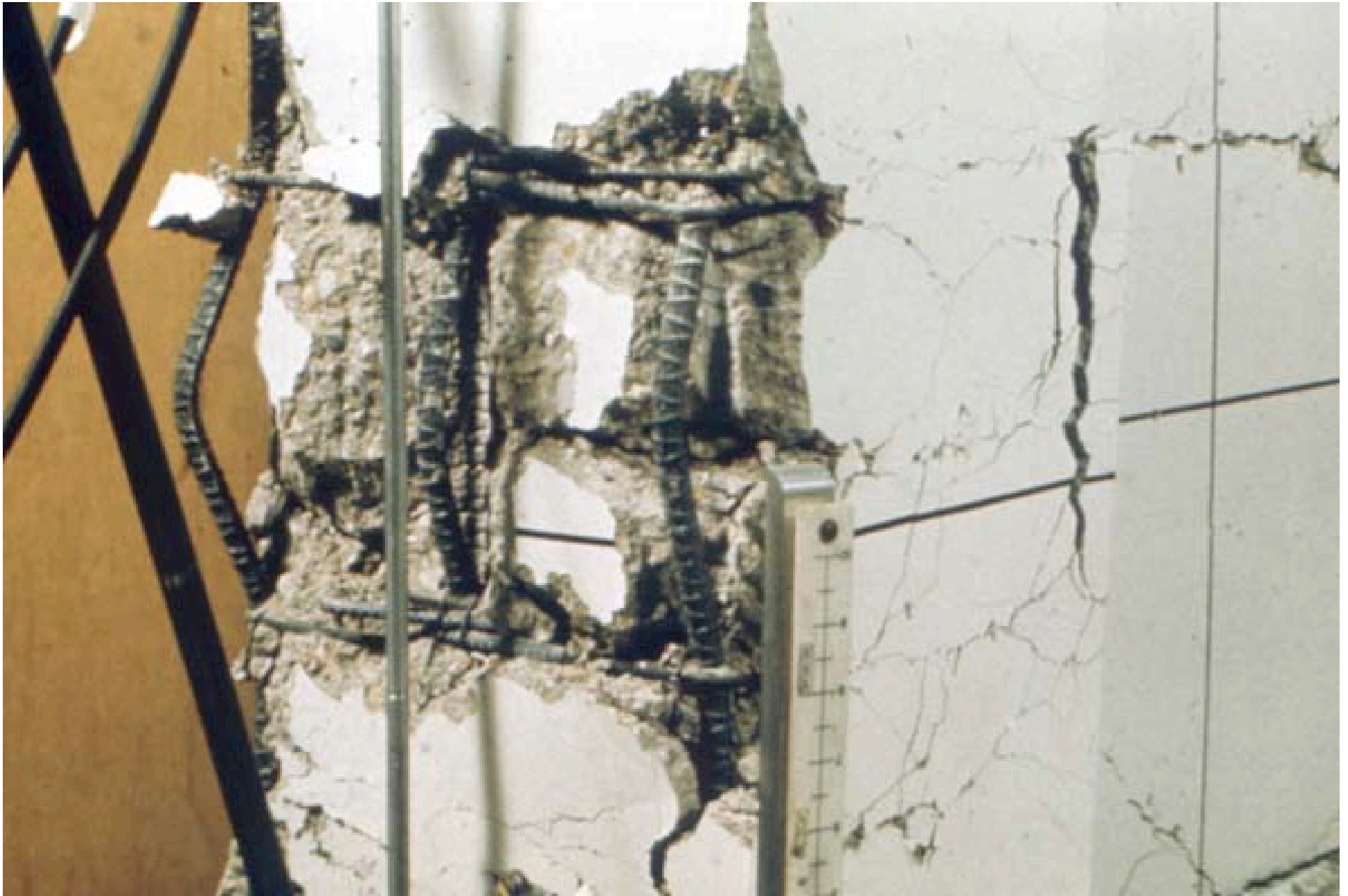
Buckled wall reinforcement
