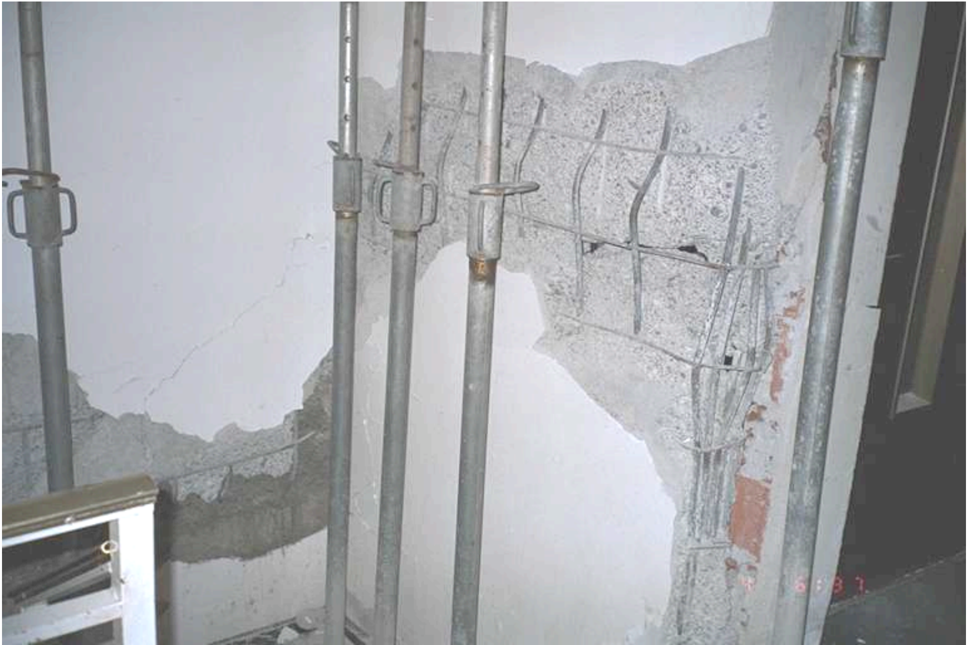
Buckled wall reinforcement -- RC1E
