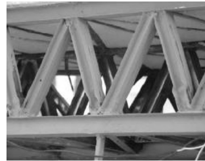
Fig. 5. Bulking of the truss member
