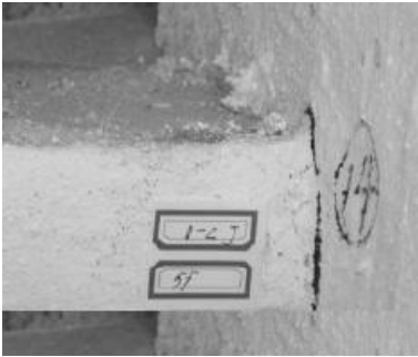
Fig. 3. Cracks of the connecting beam at 5th floor
