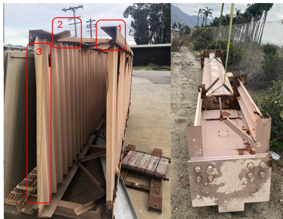
Figure 5.1: The box beam and post separated during removal of the Seacliff sign structure from its location
