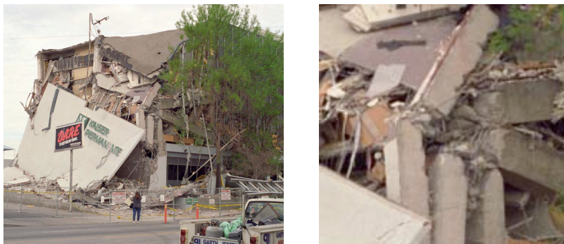
(a) Kaiser Permanente Building, Northridge earthquake, 1994 (photo courtesy of G. Edstrom)
