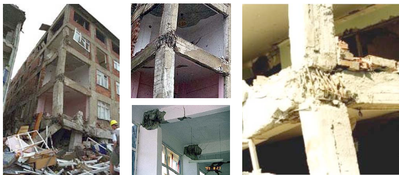
(b) A Building in Turkey, Izmit earthquake, 1999 (Sezen et al. 2000, Engindeniz 2008)
