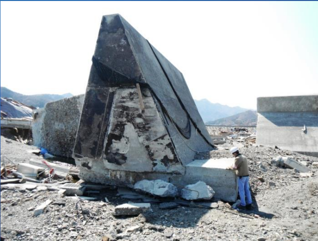
Large displaced seawall segment
