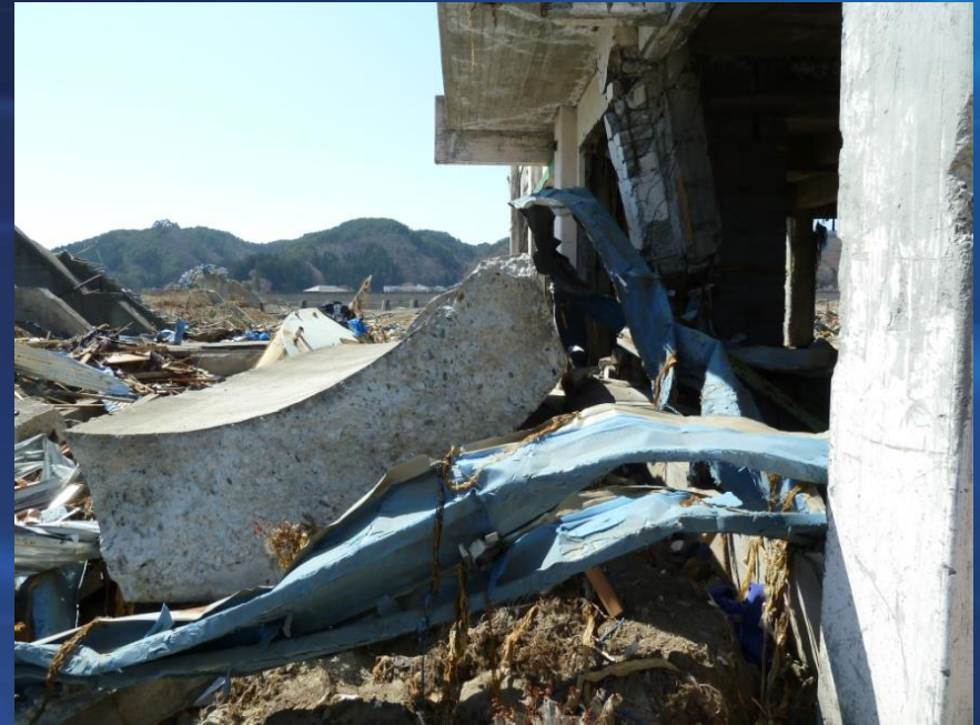
Segment of failed seawall impacted and damaged a concrete column in Tarou
