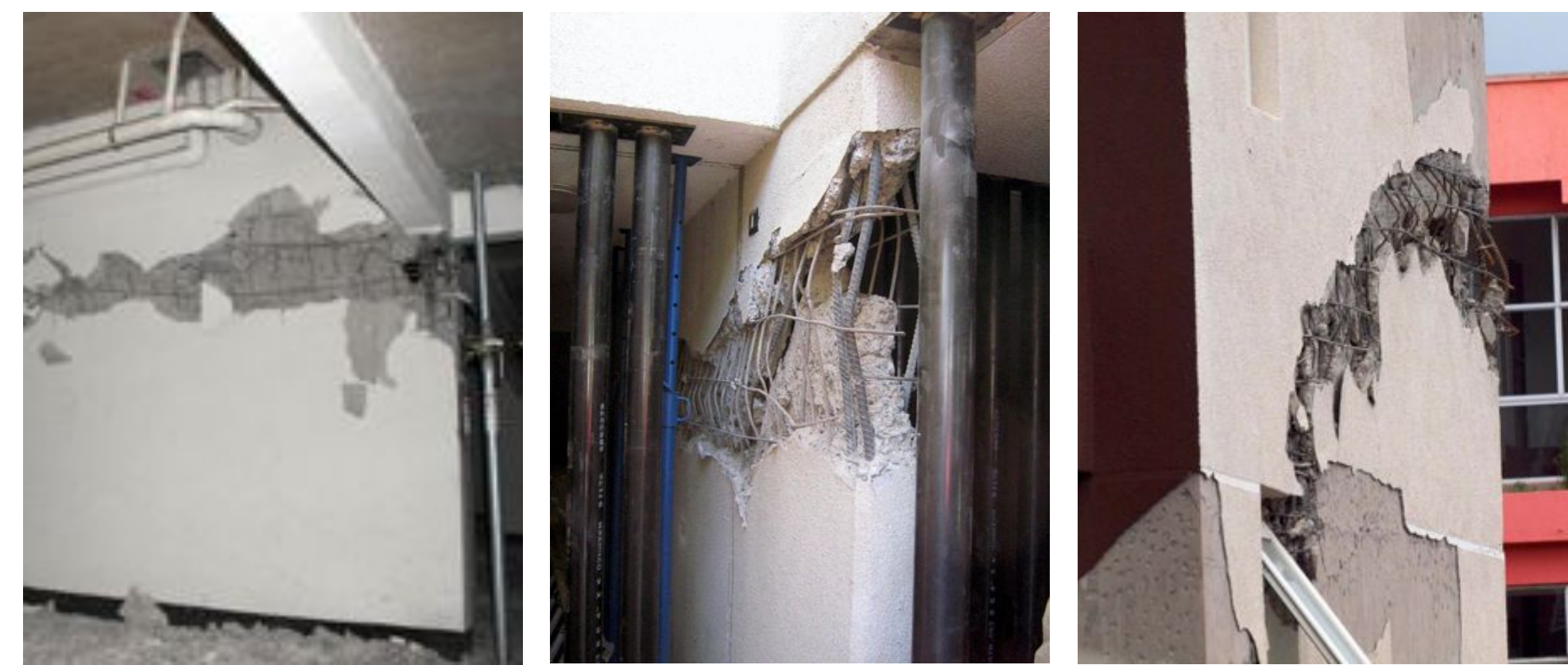
Figure 1. Buckling of Longitudinal Bars of Shear Wall with NSBE
