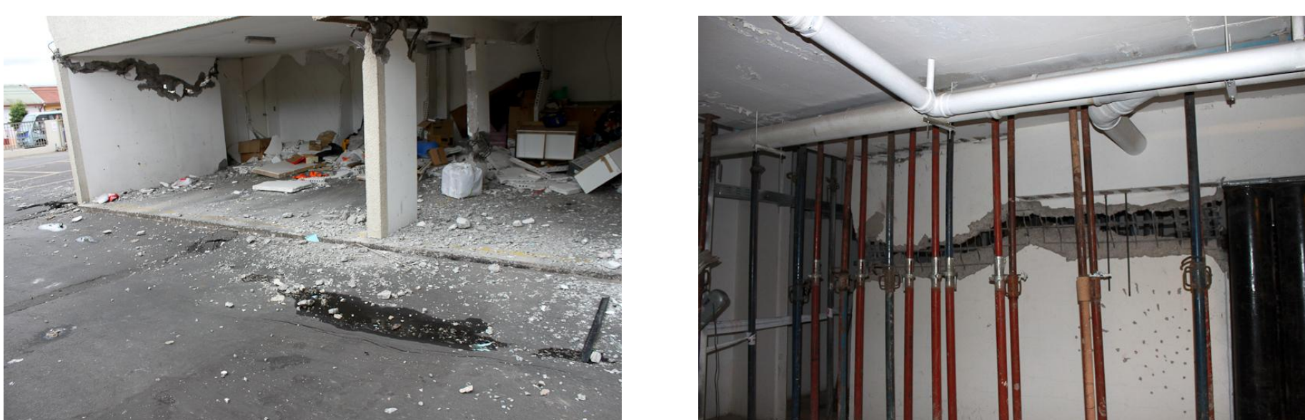
Figure 3 & 4: Typical damage seen in shear walls after February earthquake
