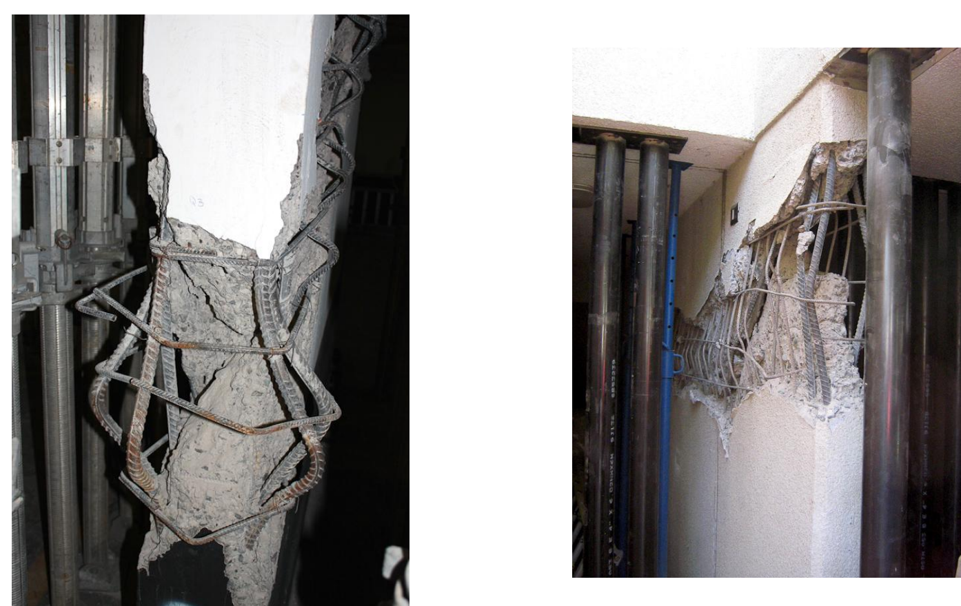
Figure 1 & 2: Failure of shear walls after Chilean earthquake
